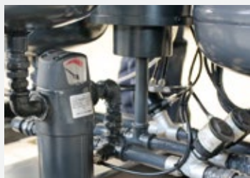
Air Filter - Pic. 4
